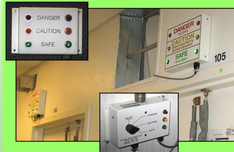
ENTRYWAY WARNING LIGHTS
